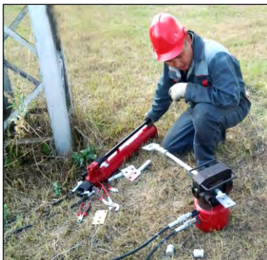
In photo PN100 in operation
