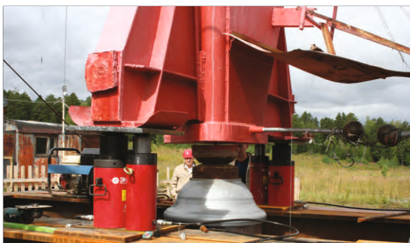
The rise of the phone tower and its holding when replacing the insulator
